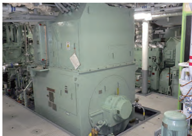
軸発電機 (水冷式) Shaft Generator (water-cooled)
