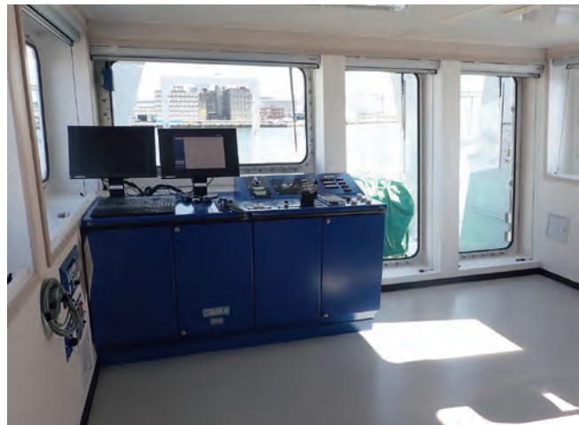
Winch&ROV制御室 Winch&ROV Control room
